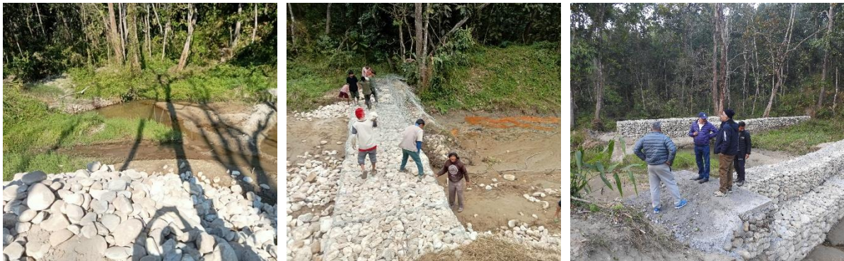
Figure 27: Photos of check dam construction before (left), during (middle), and after (right)
