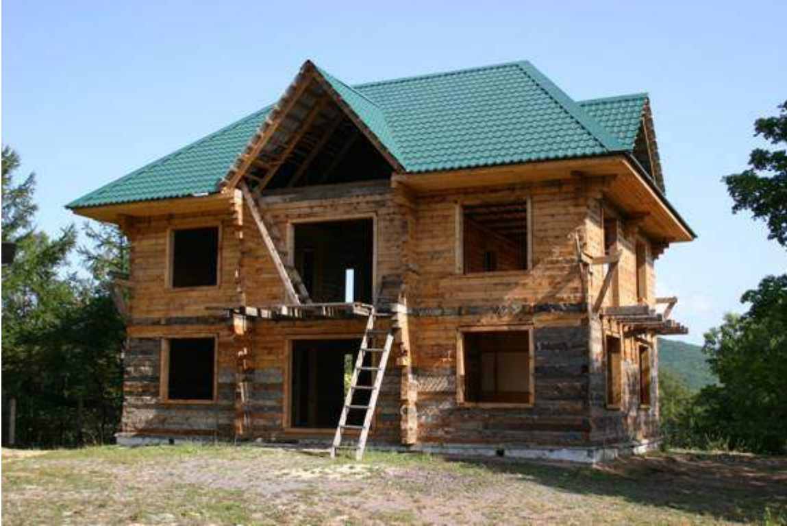
Photo 4. Office and graduate student housing under construction in Terney, September 2005. Photo by J. Goodrich/WCS.
